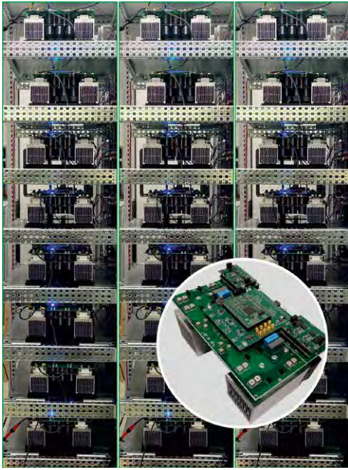
500 kVA - 9 levels modular multilevel converter (MMC)
